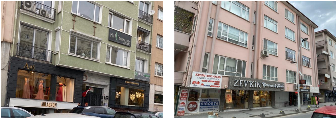
Figure 2: Examples of the removal of infill walls due to the conversion of basement floors into shops (from Esra Bostancıoğlu archive, Adapazarı).
