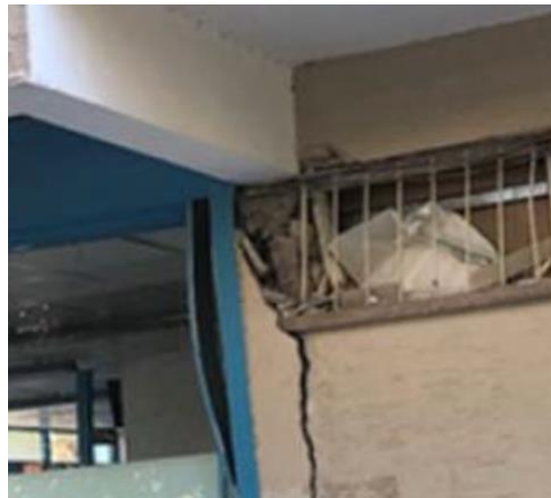
Figure 5: Damage to band windows in a building during the 2020 Izmir Earthquake (IMO, 2020).
