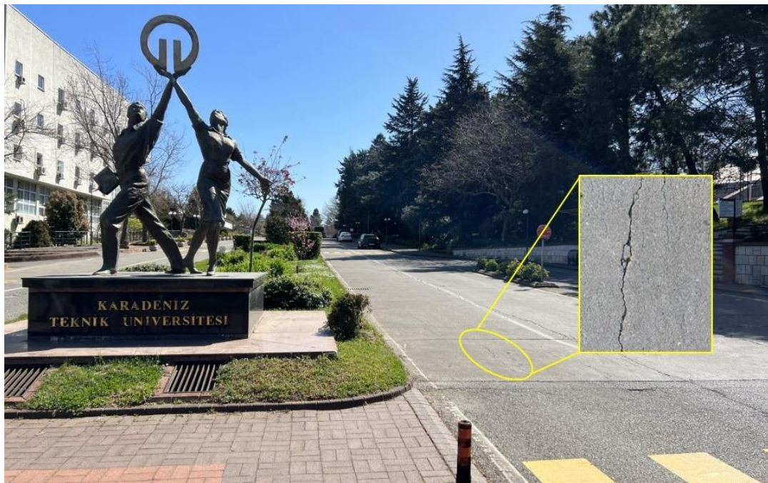
Figure 2: Sampling of crack images obtained from the roads in Karadeniz Technical University Campus.
