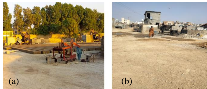
Figure 3: Site Visit (a) solid block manufacturing yard (b) hollow blocks manufacturing yard.
